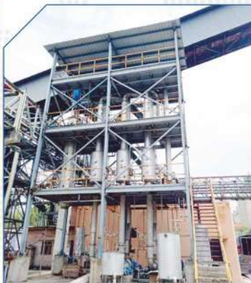
ACC CEMENT 60 KLD
