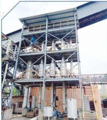
ACC CEMENT 60 KLD
