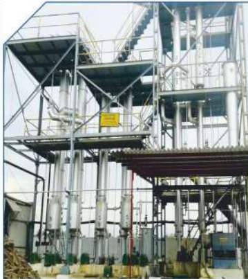
ANGERIPALAYAM CETP PVT LTD - 200 KLD
